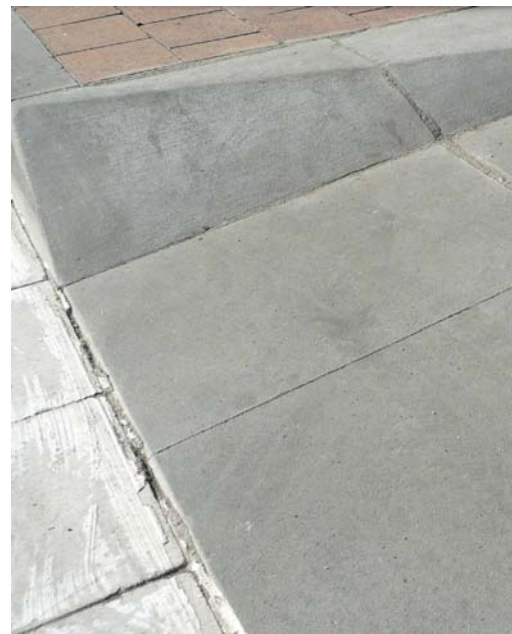
Foto Inferior. Granollers. VADO PEATONAL V57pg Bottom Photo. Granollers. V57vg PEDESTRIAN DROPPED KERB
